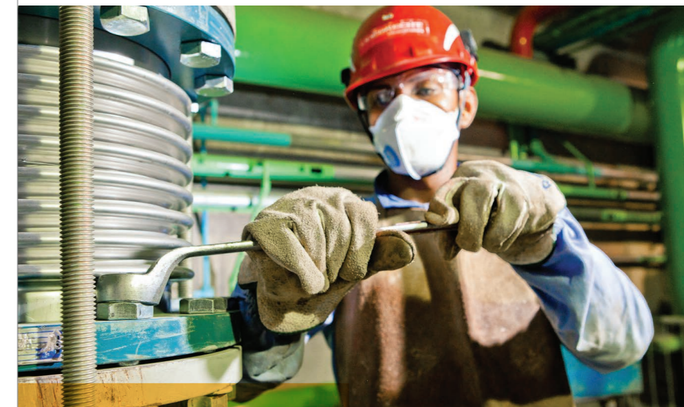
Santo Antonio Hydroelectric Plant, Rondonia – Brasil
